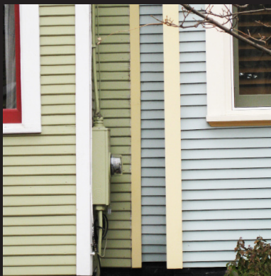
Example of an electric meter that has been appropriately painted to match the adjacent facade.
