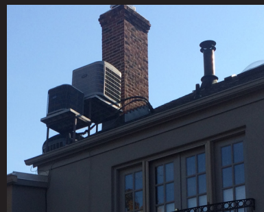
Example of inappropriate unscreened roof-mounted HVAC.
