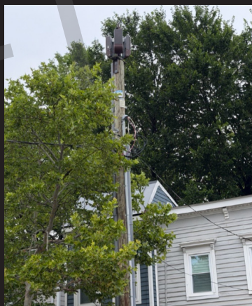
This is an example of a small cell pole installed in the public right-of-way.
